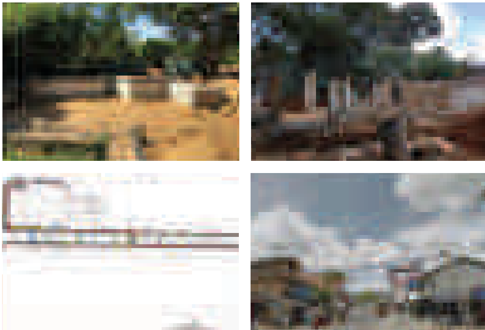
Redevelopment of SLBC Open Air Theater Redevelopment of Surapura Open Air Theater Landscaping of Dharmapala Mawatha
