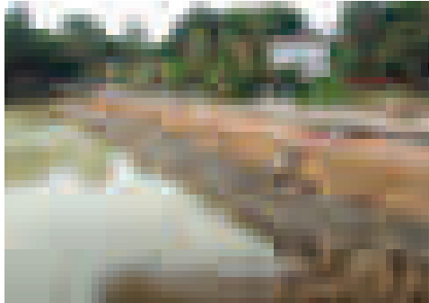
Rehabilitation of Two Pilot Ponds in Jaffna (Pilliyar Kovil Kulam ) ( In Progress)
