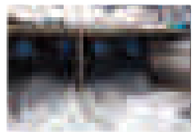
NLPS pumps at testing for June 2021 rain
