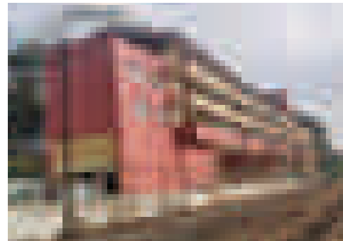
Construction of 4 storied building for relocation of part of workshops and office spaces of Sri Lanka Railway in Kandy
