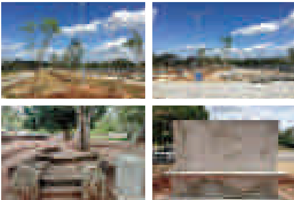
Redevelopment of Sri Maha Bodiya Eastern Entrance Vehicle Park and Erection of Interpretation Boards in Sacred City
